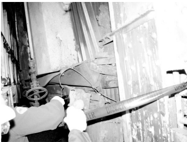
9.3 Inspecting details of boiler explosion, Dearborn, Michigan, USA
